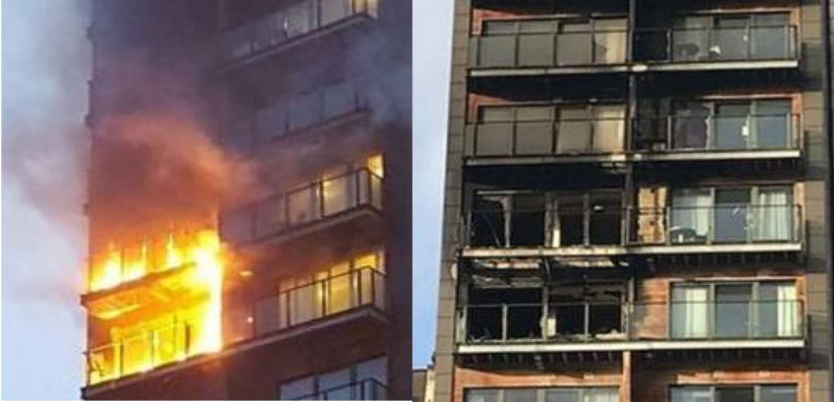
Photos showing the rapid spread of fire due to combustible privacy screen and decking, and absence of soffit.
